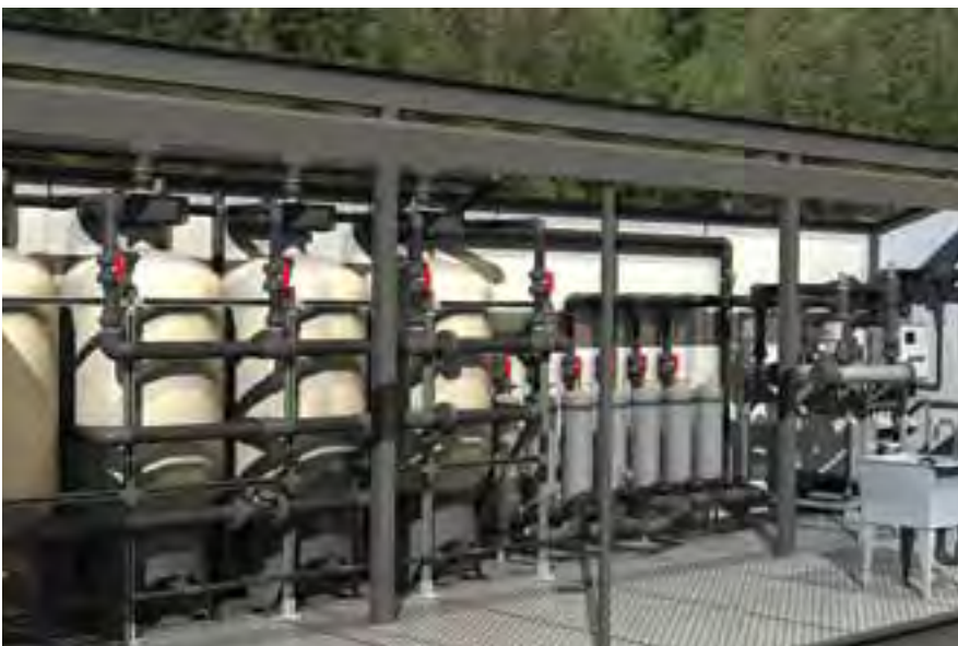
The water treatment process includes dual booster pumps, self-cleaning media filters, cartridge filters, ultraviolet primary disinfection and residual chlorination.
